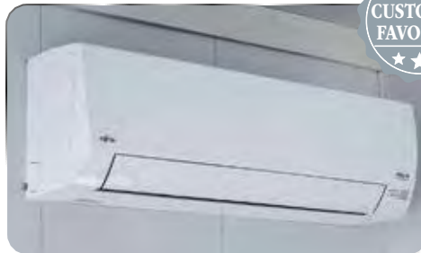
Interior View of MINI SPLIT HEATER/AC UNIT
